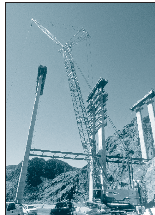
The Manitowac 2250 crane is located on the Nevada side of the bridge and is being used to construct pier caps and columns.
