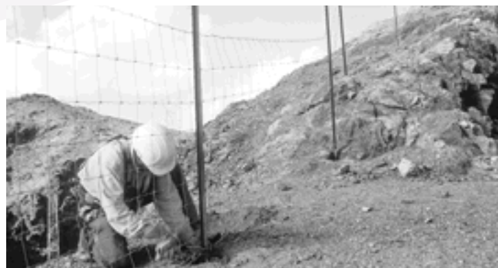
Wildlife and tortoise barrier fencing is installed in designated areas on the project to prevent wildlife from entering the work area.
